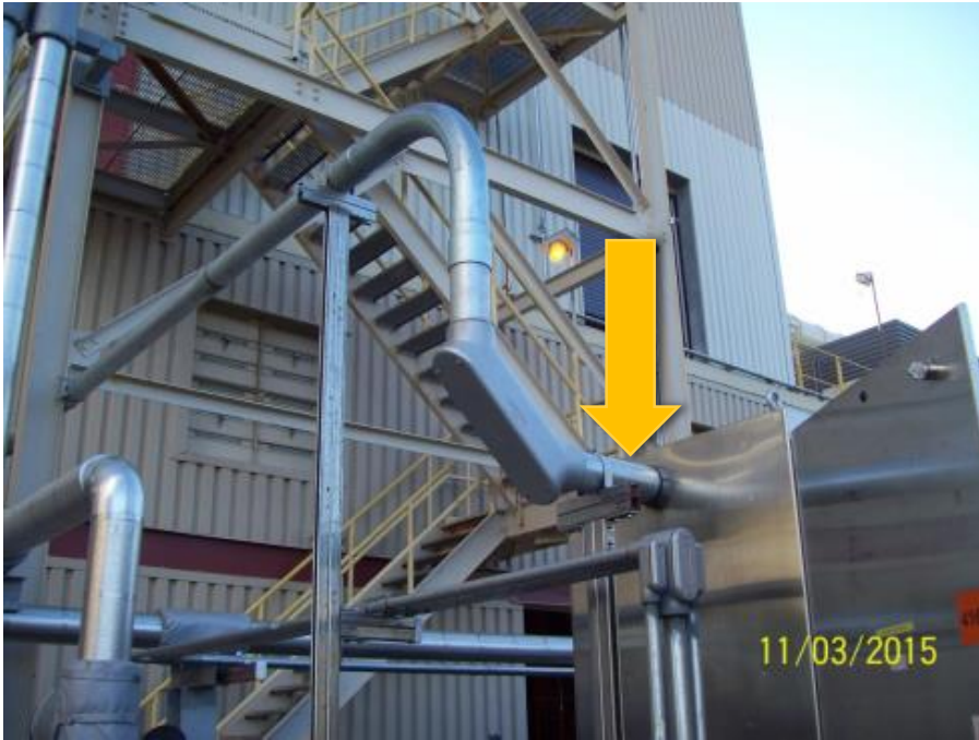
Single conduit feed for (2) circuit, 2MW 4160V
