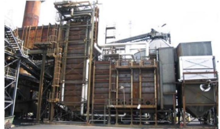
Port Arthur Steam Energy/Oxbow Corp, Texas
