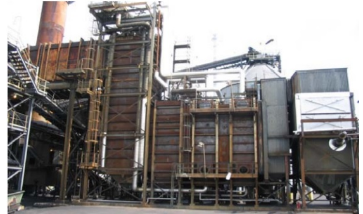
Port Arthur Steam Energy/Oxbow Corp, Texas
