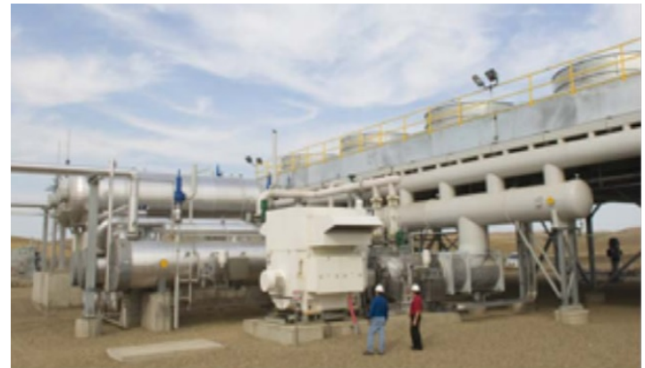
Northern Boarder Pipeline, North Dakota
