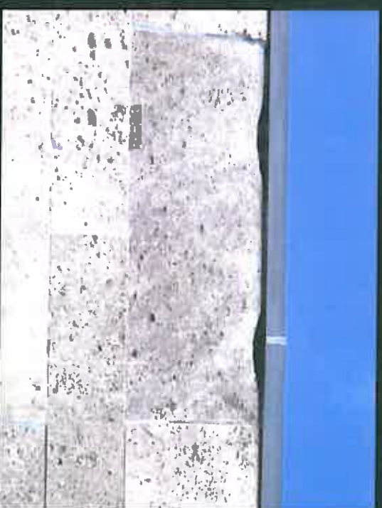
Photo 2: Spall in stone veneer at parapet coping
