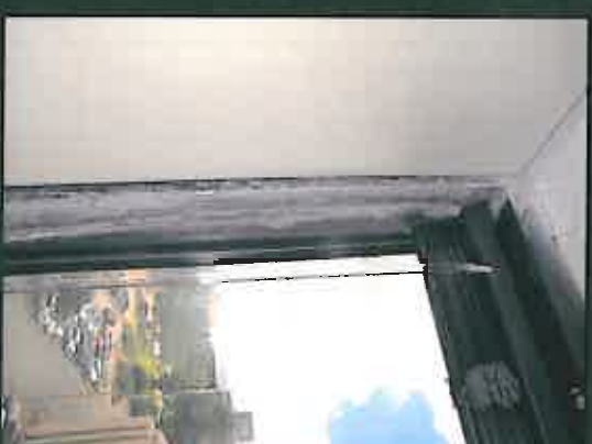
Photo 2: Moisture staining on window framing
