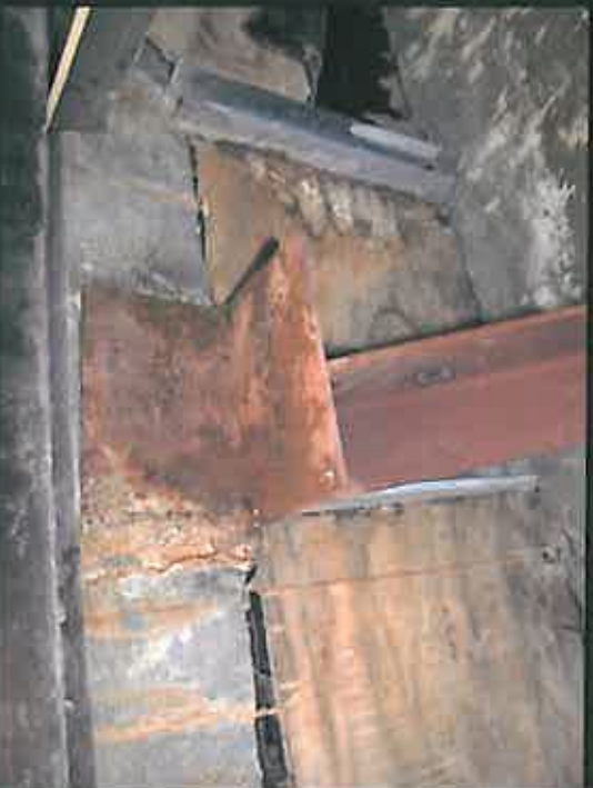
Photo 3: Corroded steel angles (above windows)
