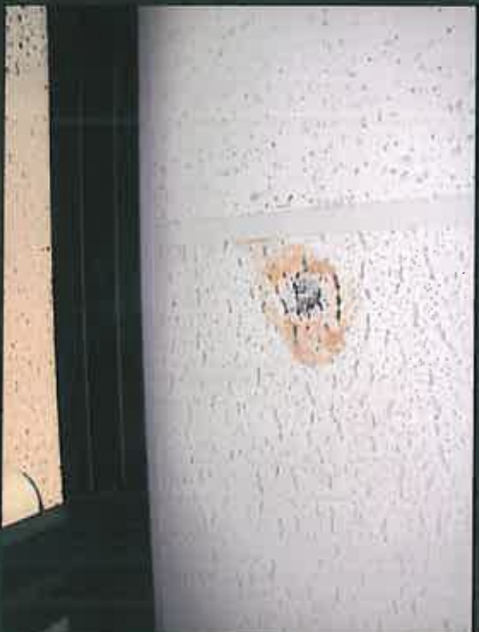
Photo 1: Water-stained ceiling tiles
