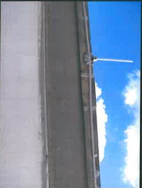
Photo 3: Distressed parapet wall coping
