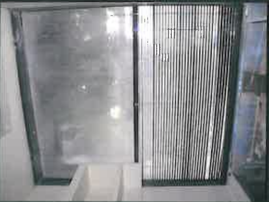
Photo 1: Moisture between window panes
