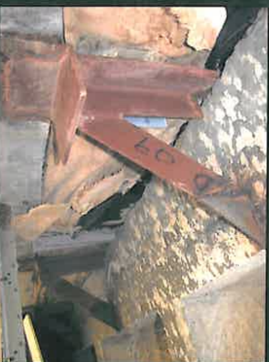
Photo 2: Deteriorated Sheathing (above windows)
