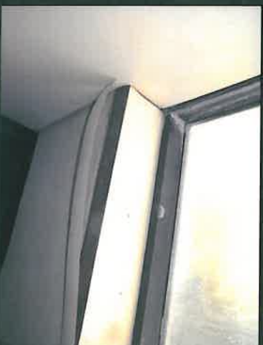
Photo 4: Delaminated vinyl below window sill
