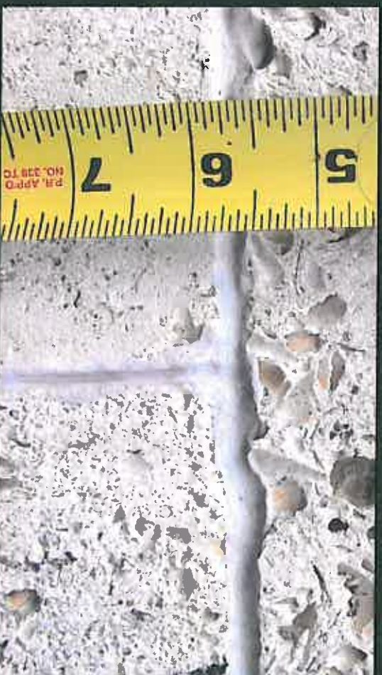
Photo 3: Deteriorated stone-to-stone joint sealant
