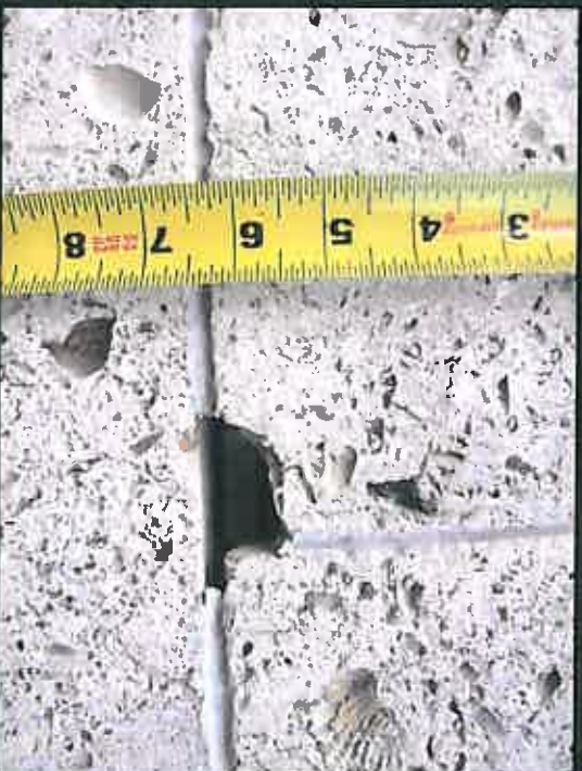
Photo 1: Typical spall in stone veneer
