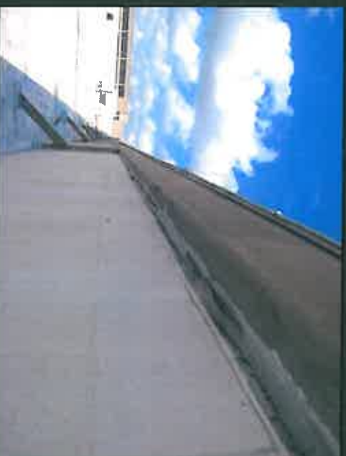
Photo 4: Failed joint sealant below parapet framing
