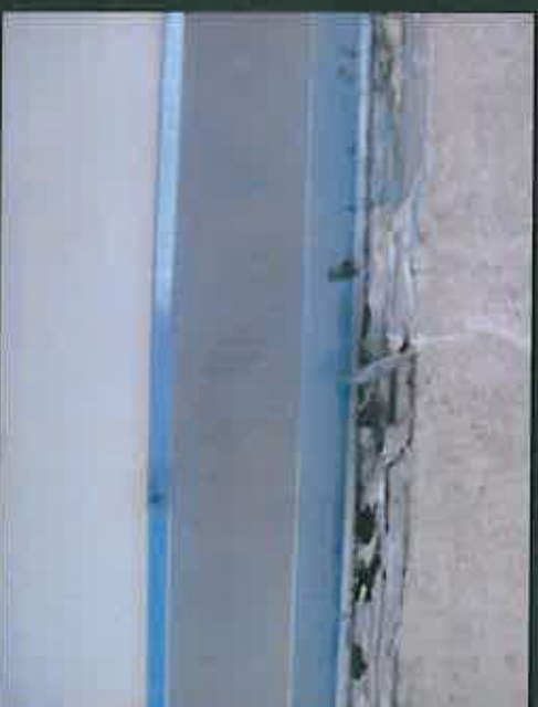
Photo 2: Failed sealant above metal flashing
