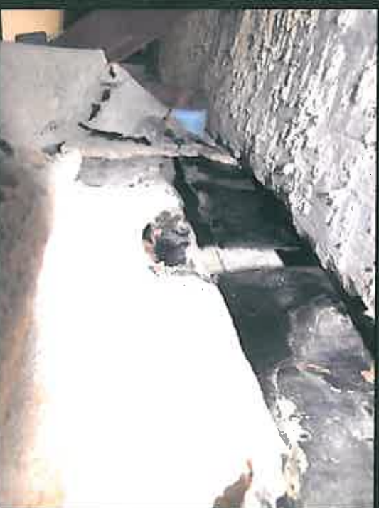
Photo 4: Damp-proofing not properly lapped
