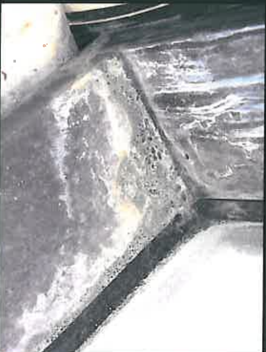
Photo 3: Moisture staining on window framing
