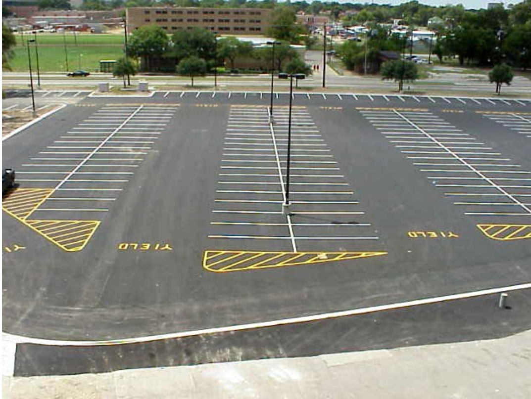
FIGURE 1.1 OVERVIEW OF PARKING LOT AND LIGHTING
