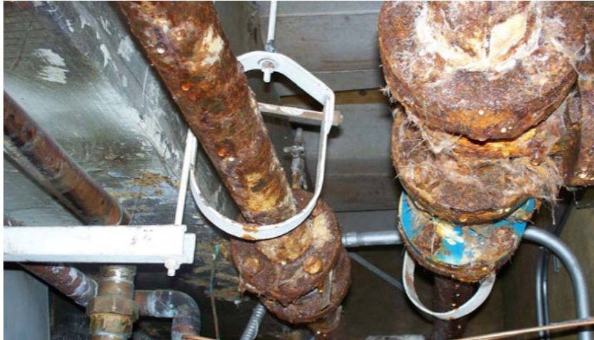
Hot Water Piping
