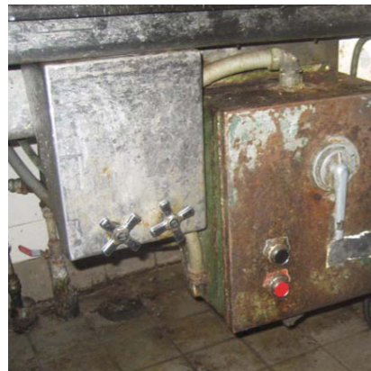
E11: Equipment showing excessive corrosion damage.
