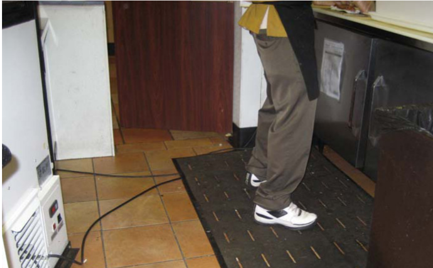
E13: Flexible cords used in violation of NEC-400.8.
