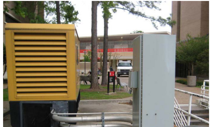
E16: Emergency Generator and ATS at UC Satellite.
