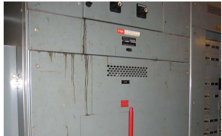
E2: Main Switchboard Main Disconnecting Means
