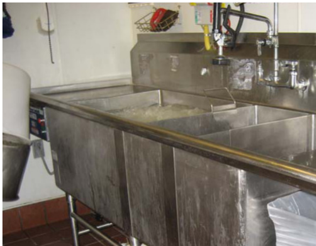
E12: Receptacles without discernible ground fault protection within 6 feet of sink.
