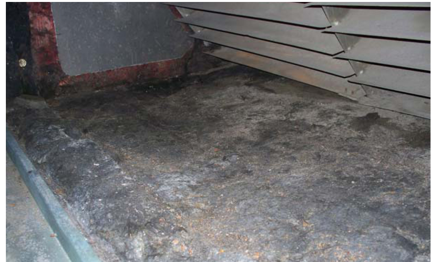
M1: Fraying ductliner
