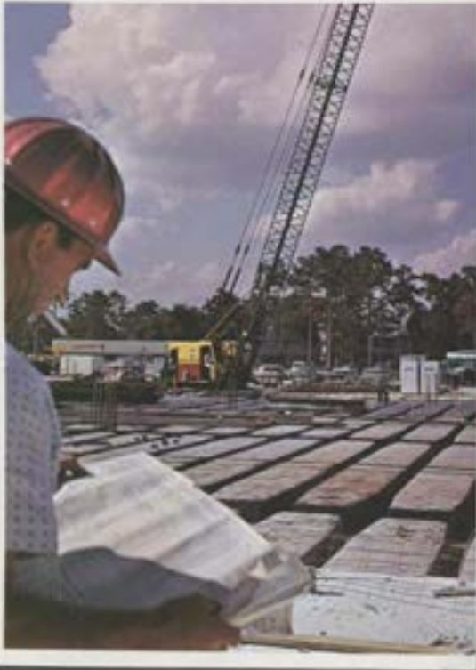
A workman checks the construction schedule as work continues on the two year project.
